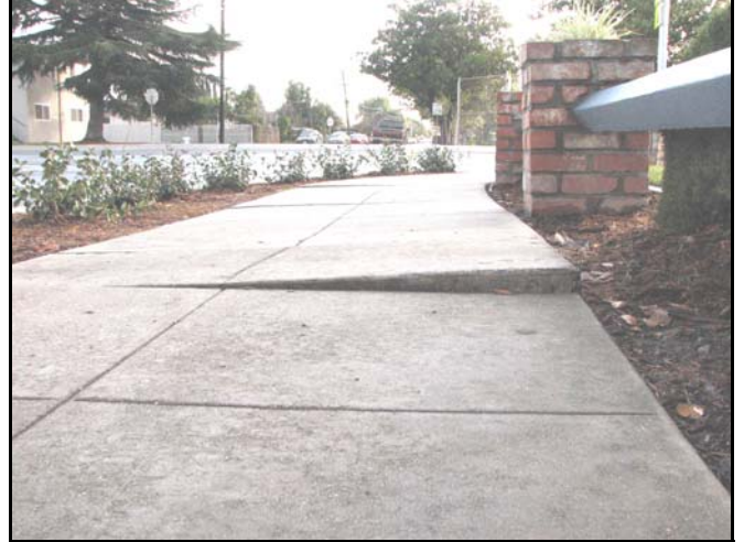
The "kids-eye view" of a sidewalk in need of repair, on Bayview Avenue near Maude.
